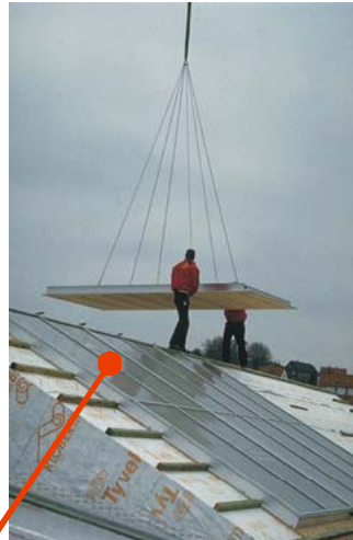
64 m 2 Solar Roof
